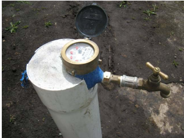
Typical metered spigot on concrete pedestal
