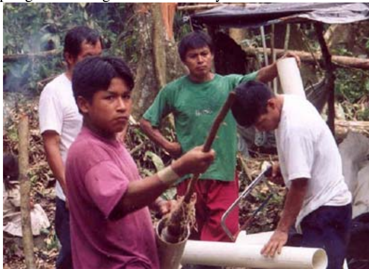
Figure no. 3 – Picture of field slotting of pipe and cleaning out the cuttings.
